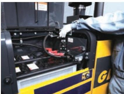
Battery main switch
